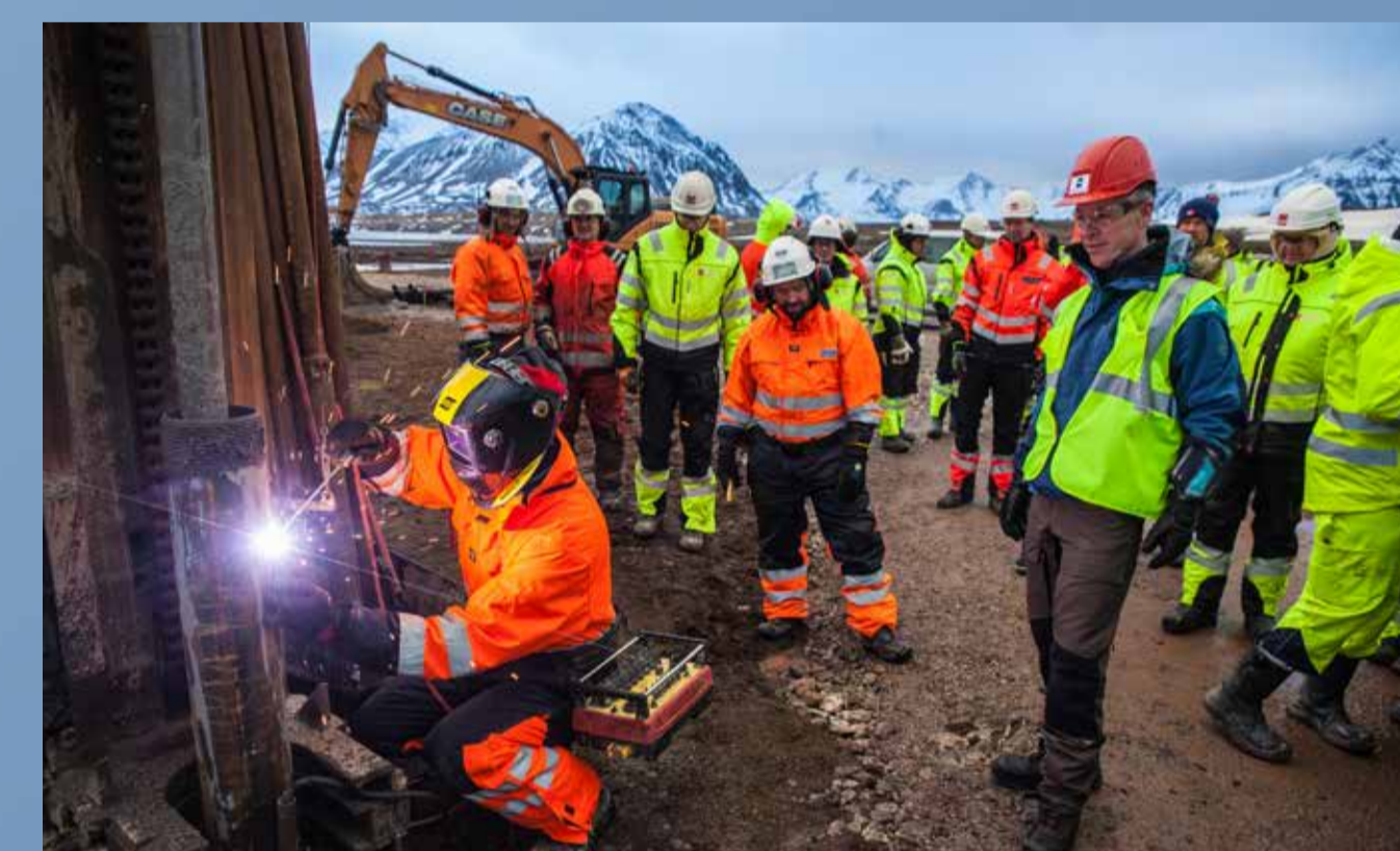
The Norwegian Mapping Authority's new geodetic Earth observatory is under way after the first pile was driven in the autumn of 2014. Performed by Jan Tore Sanner, Norway's Minister of Local Government and Modernisation, that ceremony marked the start of building work.
