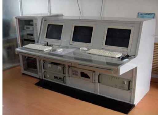
New operation console
