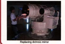
Replacing dichroic mirror
