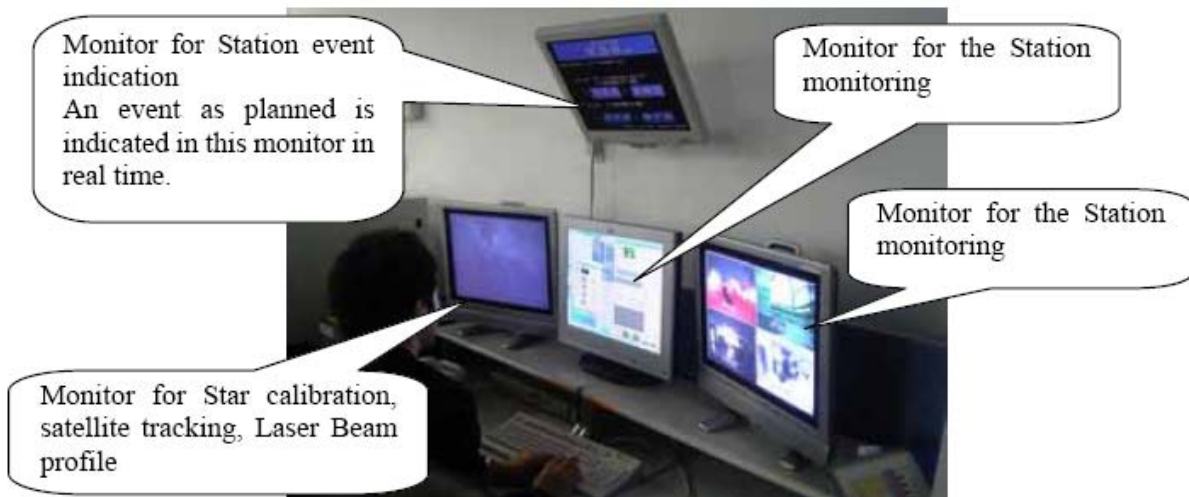
Fig.2 Station control system in Tsukuba
