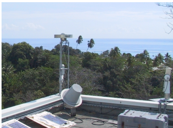
Fig. 4: the THTI GPS antenna on the roof
