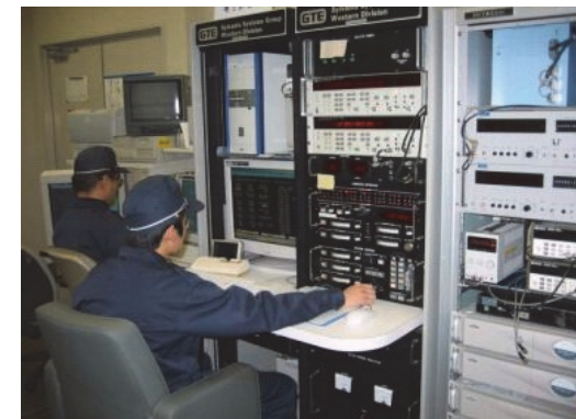
Control & monitor devices
