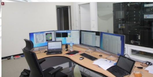
Operation & Electric Room
