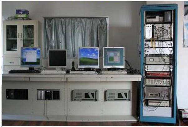
Ranging control room
