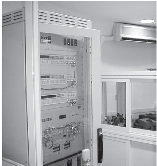
Figure B-54. New rack configuration.
